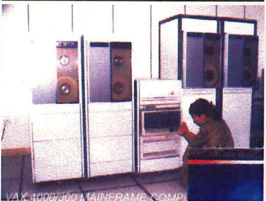
NATIONAL DATA CENTRE PUNE
